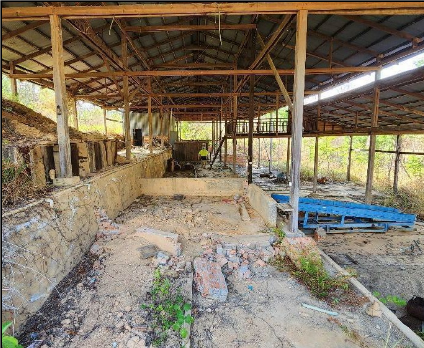
Figure 7: Gold Metals Group's ore treatment plant in 2024 at the Camp Prospect. The plant was closed down in approximately 2020 by the Cambodian Government and now lies in ruin.
